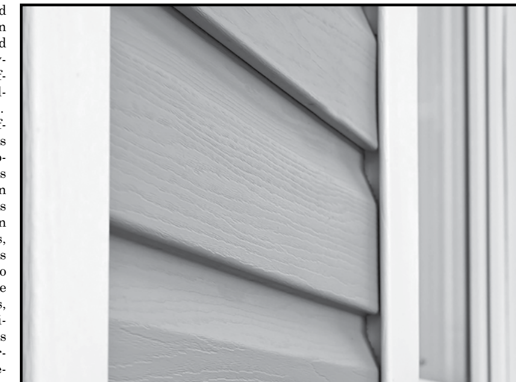
Mildew can grow on home siding as well as fences and other exterior structures.
